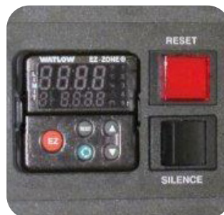
Redundant Process Temperature High Limit (Standard)
